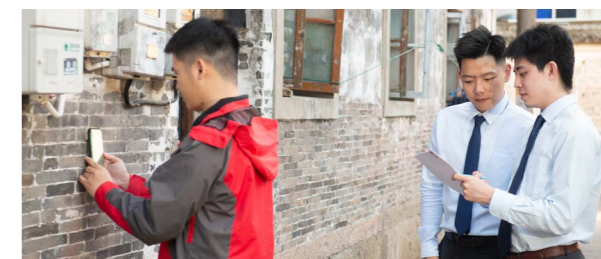
The personnel of the Ningbo Branch prevented a falling incident caused by the hollowing of the external wall by measuring and recording the cracks and hollowing of the external wall, guaranteeing the property safety and life safety of residents
